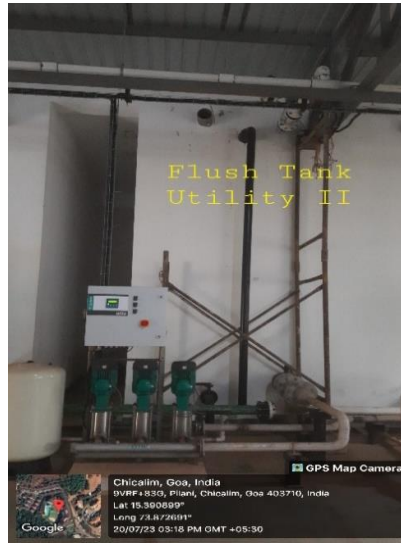
Flush Tank Utility-II
