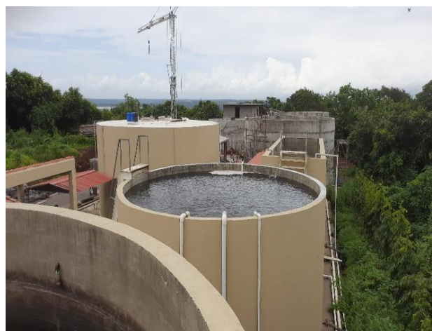
SBR tank system
