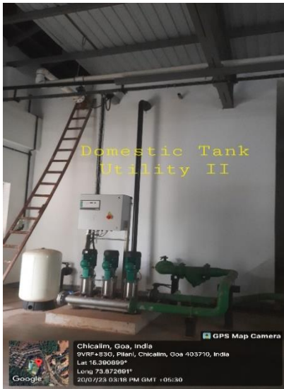
Domestic Tank Utility-II
