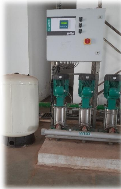
UTILITY II FLUSH PUMPS
