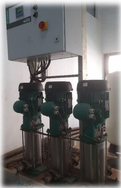
Utility-I Domestic Pumps
