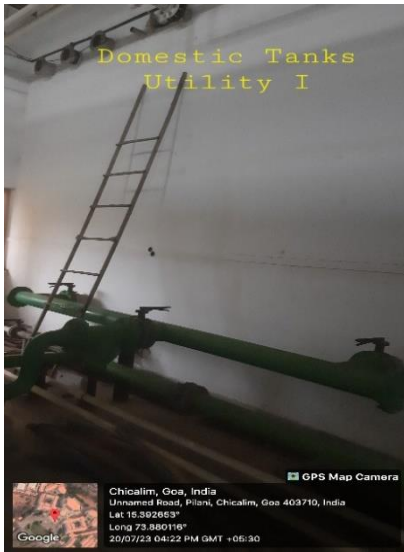
Domestic Tank Utility-I
