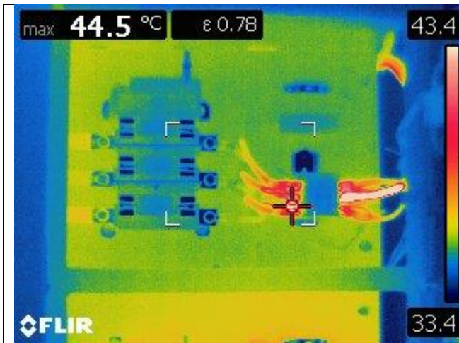
(ii). Thermal Image of Capacitor bank Feeder (8F6) (50 kVAR) at PCC-2
