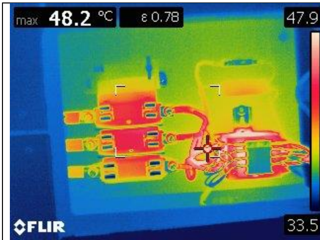
(vi). Thermal Image of Capacitor bank Feeder (8F4) (15 kVAR) at PCC-2
