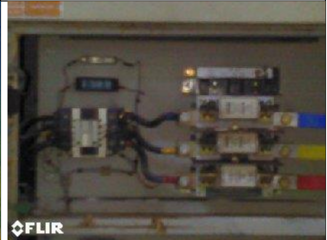
Normal Image of Capacitor Bank Feeder (8F1) (25 kVAR) at PCC-2
