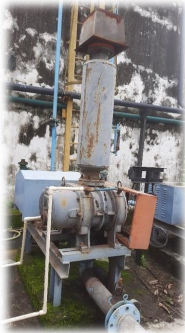
Air blower 67WC
