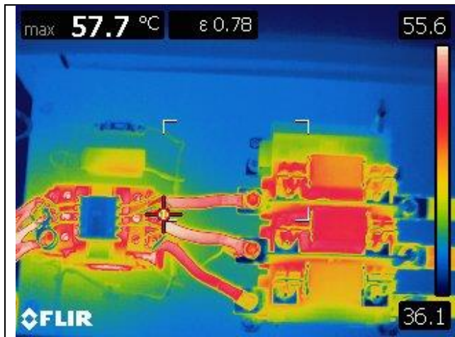
(i). Thermal Image of Capacitor bank Feeder (7F1) (50 kVAR) at PCC-2
