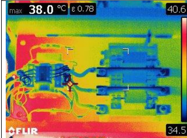
(iii). Thermal Image of Capacitor bank Feeder (8F1) (25 kVAR) at PCC-2
