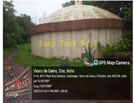
Sump Tank-III (Capacity: 4.5 L Liter)
