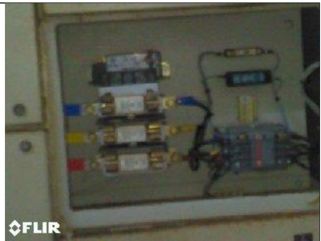
Normal Image of Capacitor Bank Feeder (8F4) (15 kVAR) at PCC-2
