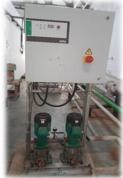
Utility-I Garden Pumps
