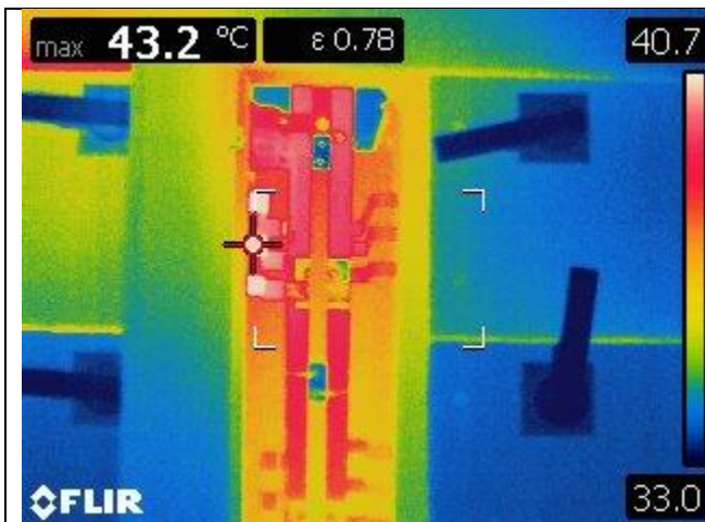
(iv). Thermal Image Busbar of PCC3 Panel
