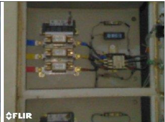
Normal Image of Capacitor Bank Feeder (8F6) (50 kVAR) at PCC-2
