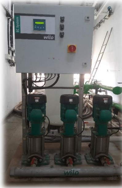
Utility-I Flush Pumps
