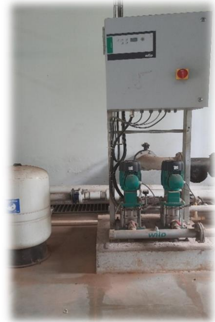
UTILITY II GARDEN PUMPS
