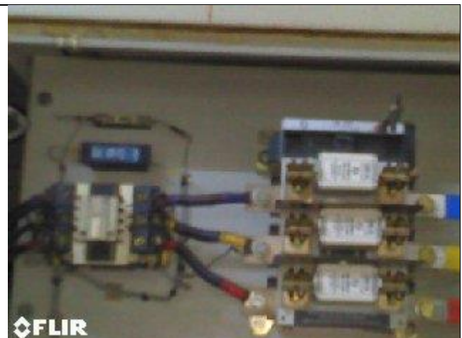
Normal Image of Capacitor Bank Feeder (7F1) (50 kVAR) at PCC-2
