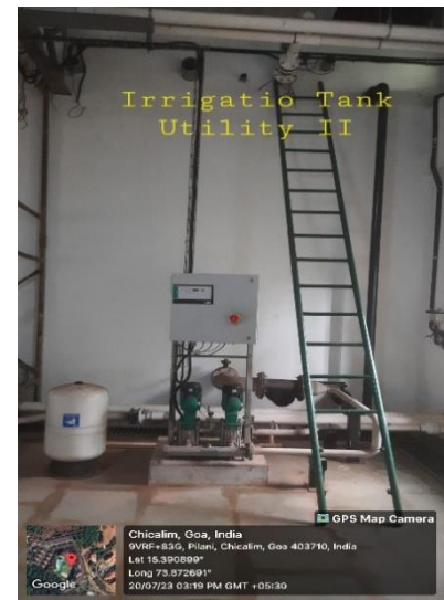
Irrigation Tank Utility-II
