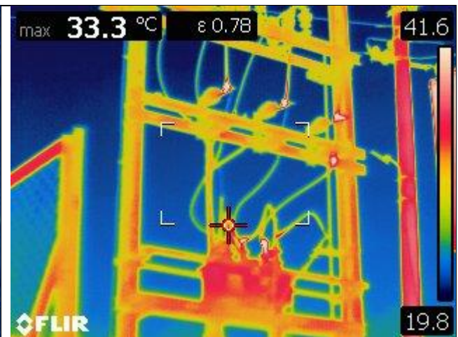
(v) Thermal Image of 2 Pole Structure at PCC2
