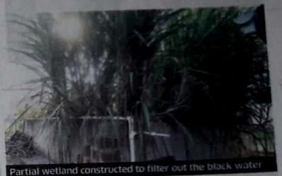
Partial wetland constructed to filter out the black water
